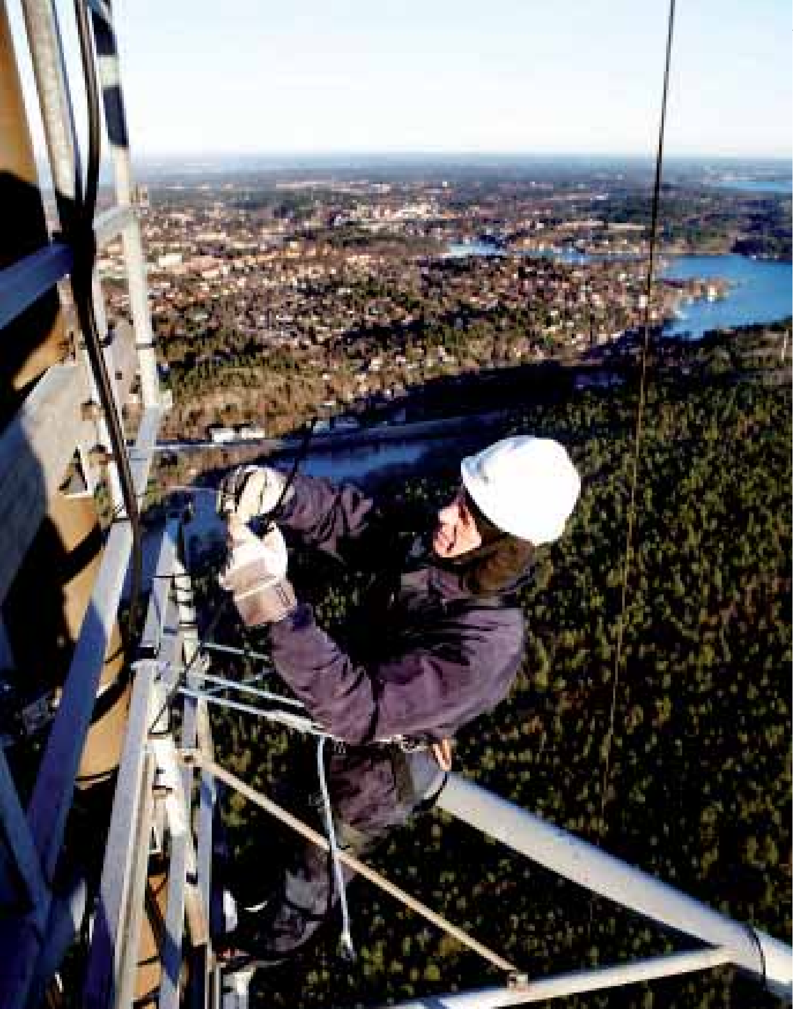
Teracom's service technicians at Nackamasten. Teracom Group owns and operates the Swedish terrestrial networks for radio and TV. The company is 100 per cent state owned. Photo: Teracom Group
