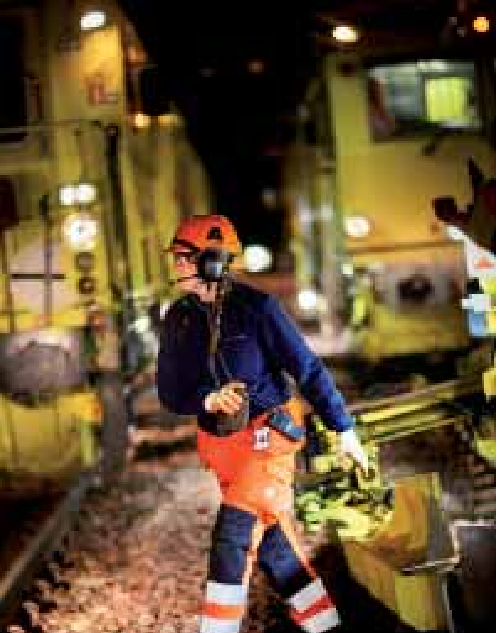
State-owned companies are well represented in the transport and infrastructure sectors. The photo depicts night work being carried out by Infranord. Photo: Infranord
